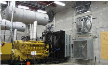
Model WPB Generator Room Exhaust
