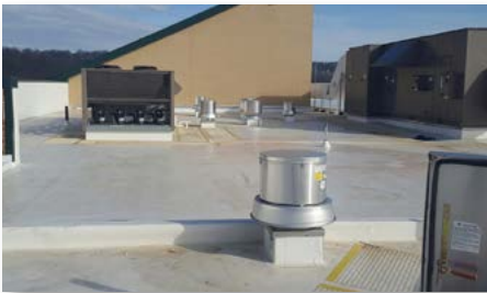
Model BCRD School - General Building Exhaust
