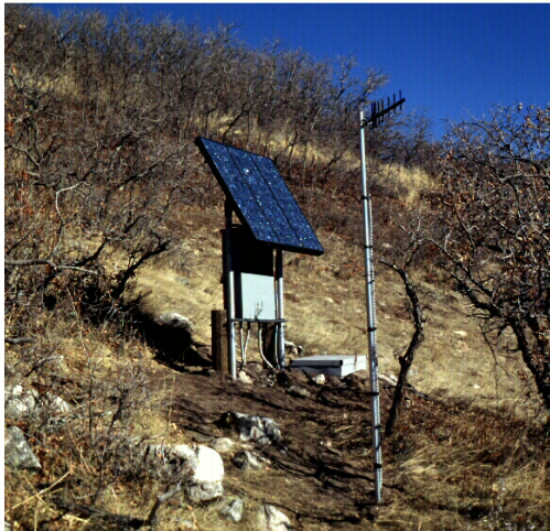
Figure 11. A solar powered GPS site with radio modem telemetry established by the University of Utah for atmospheric and geodetic applications, with assistance from UNAVCO. The site is located in a geologically stable location with a radio telemetry link to campus. The enclosure beneath the solar panel contains GPS receiver equipment and batteries. Similar installations are expected for universities interested in combined atmospheric and geodetic applications.
