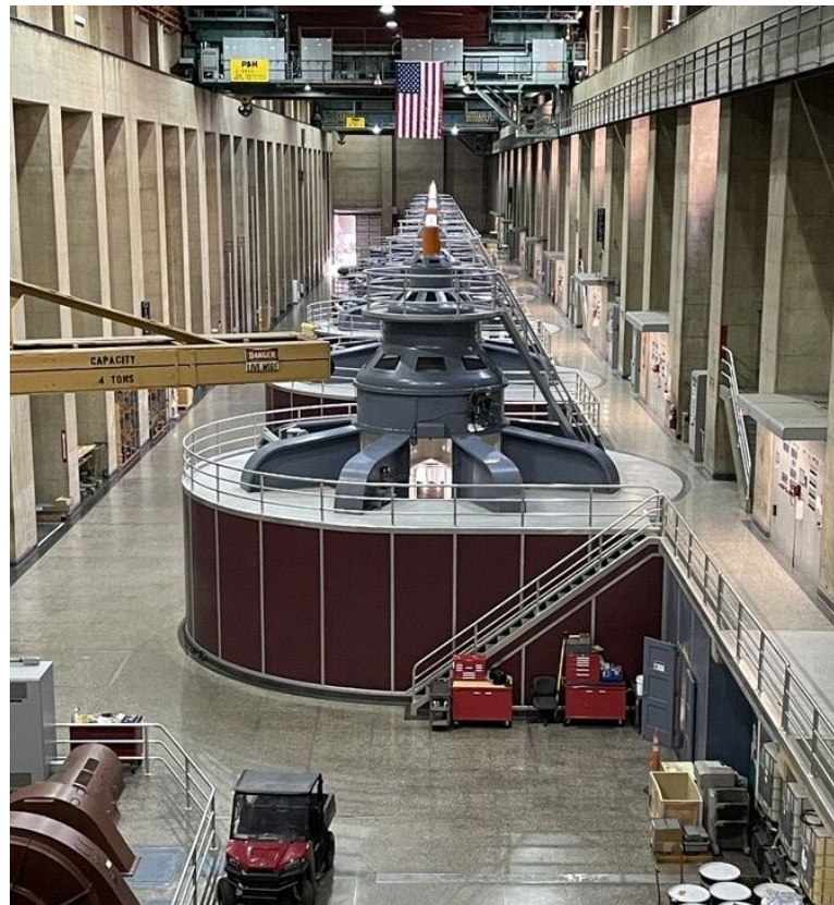
There are 17 generators in the Hoover Dam Powerplant in Nevada. When all are operating together at maximum capacity, they can produce about 2,080 megawatts—enough power for 1 million homes.
