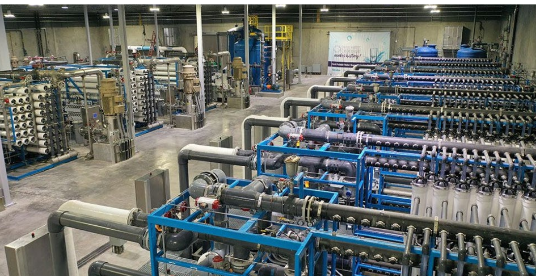
Reclamation funds numerous innovative water projects. For example, the Pure Water Oceanside facility is an advanced water purification program that purify recycled water to create a new, local source of high-quality drinking water. The facility will produce enough water to provide more than 30 percent of Oceanside, California’s water supply and reduce dependence on water from the Colorado River.
