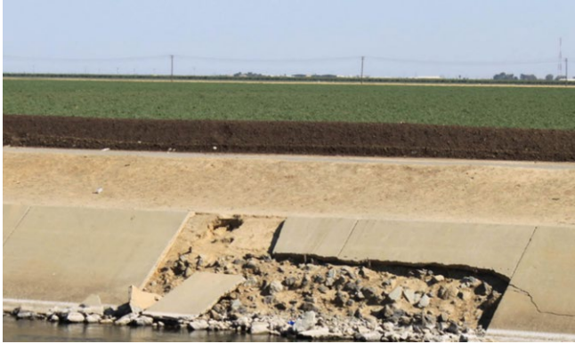
Portions of the Delta Mendota Canal have been damaged due to land subsidence resulting from over-pumping of aquifers in response to climate change-driven surface water shortages.
