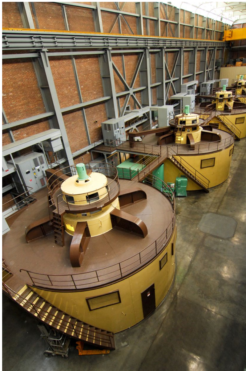
Generators inside the powerplant at Palisades Dam, Idaho.
