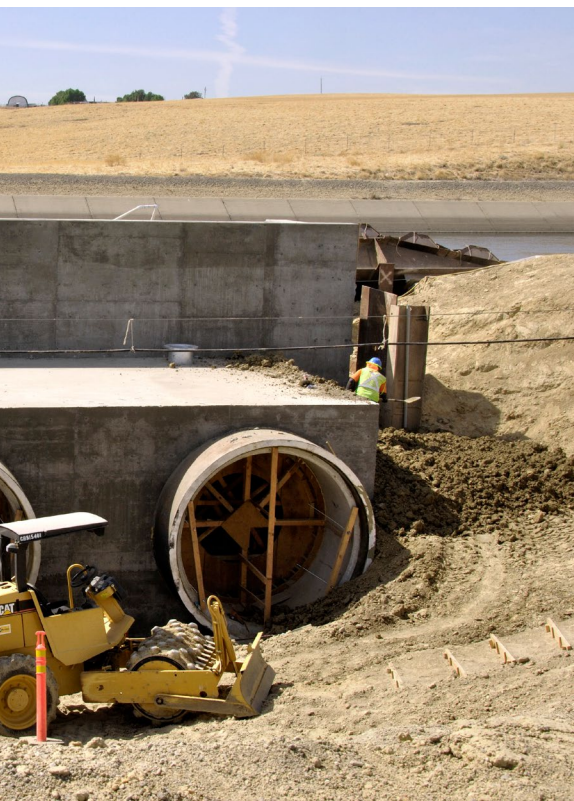
Bottom: Shows construction of the turnout at the California Aqueduct end of the Intertie Project.
