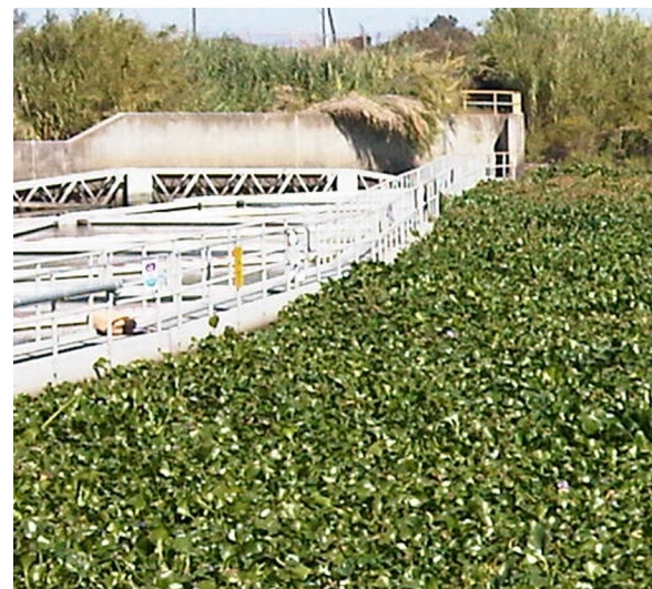
Water hyacinth spread across the intake channel for the C.W.
