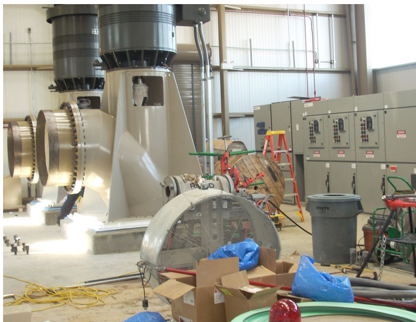
Motors and pumps are installed in the pumphouse.
