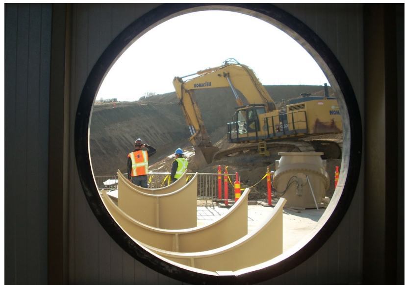
A view from inside the Intertie pump house looking out at pipe support structures.
