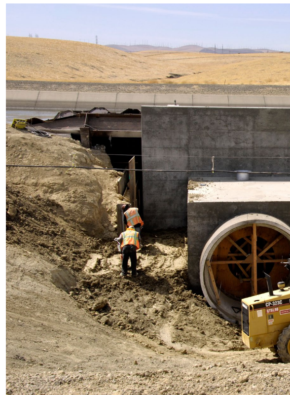
Top: Shows construction of the pump station at the Delta-Mendota Canal end of the Intertie Project.
