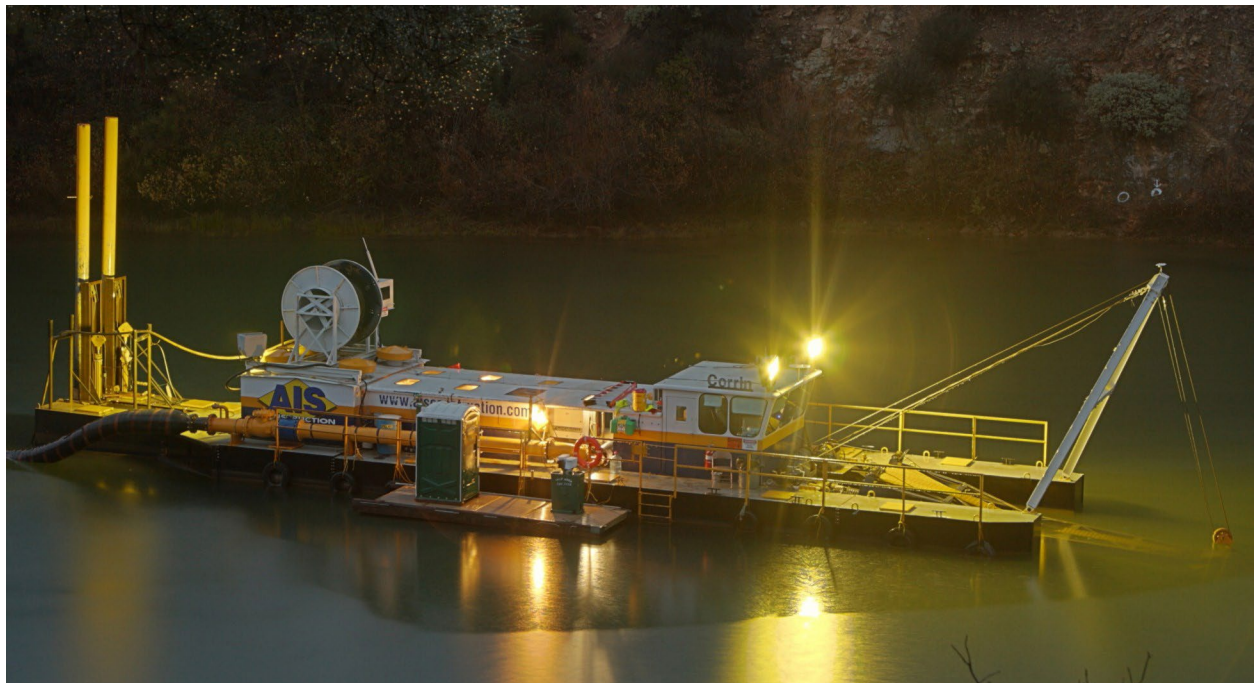
One of the Region's projects during 2011 involved removing 3,500 cubic yards of sediment from the Spring Creek Arm of Keswick Reservoir in Northern California. The sediment had blocked access for inspection of the outlet works and spillway structures of the Spring Creek Debris Dam. A dredge, shown here at night, removed the sediment.
