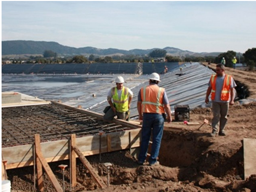
Workers construct a facility that is part of the North Bay Water Reuse Program.
