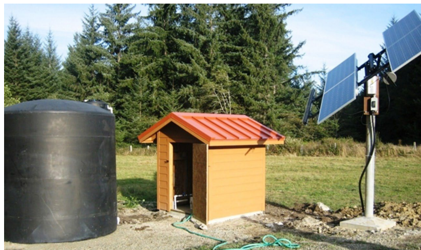
One of the new solar-powered wells constructed at the Elk Valley Rancheria in Crescent City, California.
