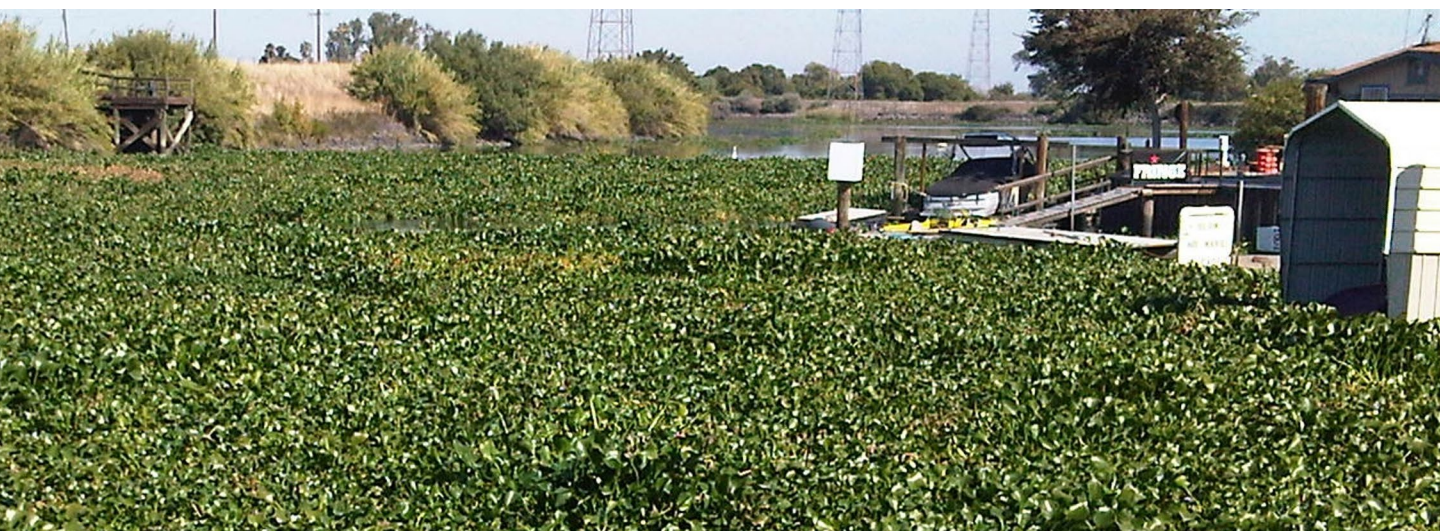
"Bill" Jones Pumping Plant in the Sacramento-San Joaquin Delta.
