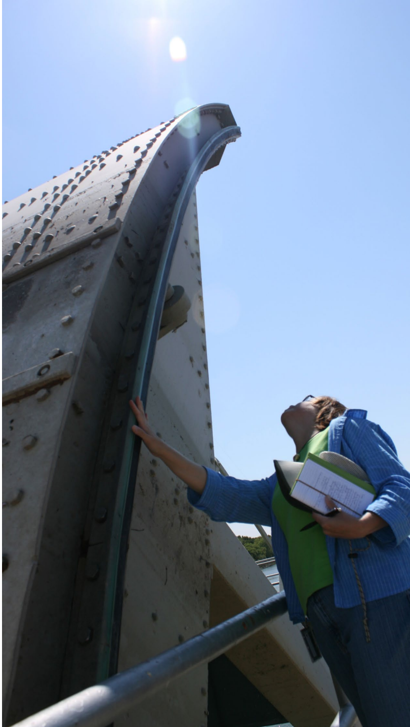
An intern looks up at radial gate on the Delta Cross Channel in this employee contest photo taken by Jeffrey Valeros.
