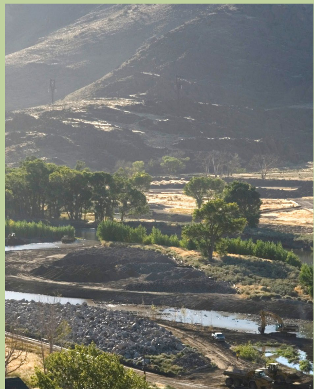
Restoration work is underway on the Truckee River in the McCarran Ranch Reserve.
