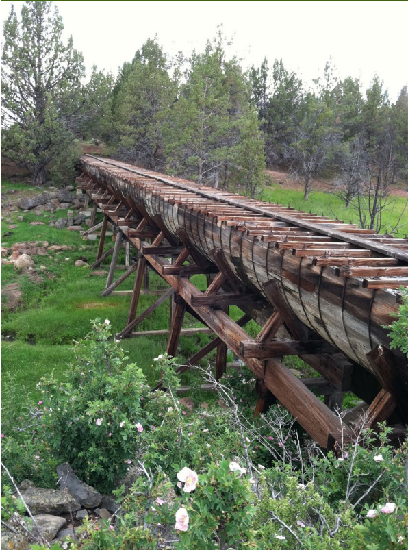
"Historic North Canal Redwood Flume (Klamath Project);" photograph by Jennifer L. Birri.
