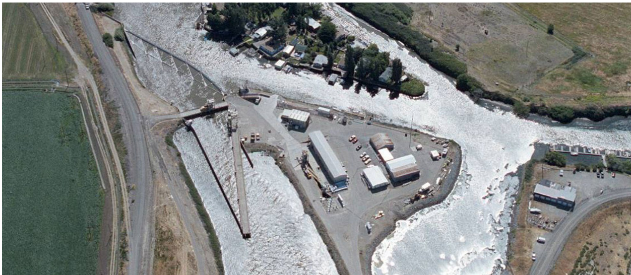
The Tracy Fish Collection Facility, near the C.W. "Bill" Jones Pumping Plant, helps protect fish.
