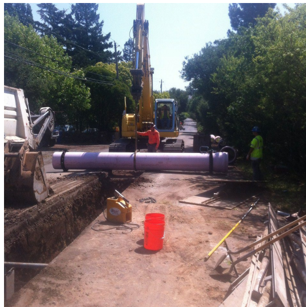
Workers install pipeline as part of the North Bay Water Reuse Program.
