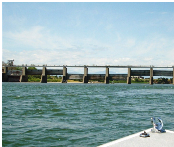
Boat heads toward the open gates of the Red Bluff Diversion Dam.
