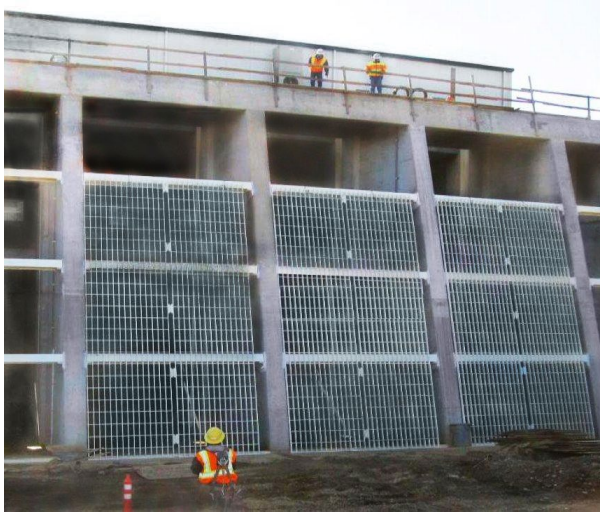
View of the screen and cleaner structure show the immense size of the project.
