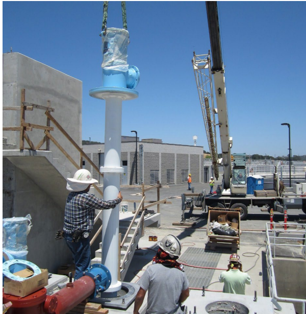
A vertical turbine pump is installed at a water reuse project near Novato, Calif.
