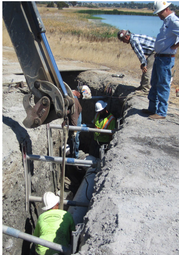
Crews put finishing touches on pipe installation at a water reuse project near Novato, Calif.
