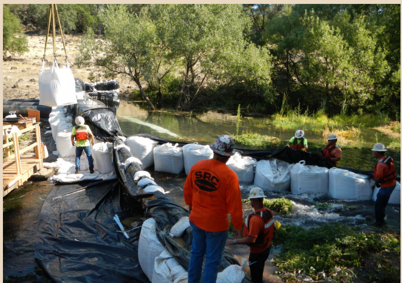
Workers use “super sacks” to build a diversion dam in Baldwin Creek.
