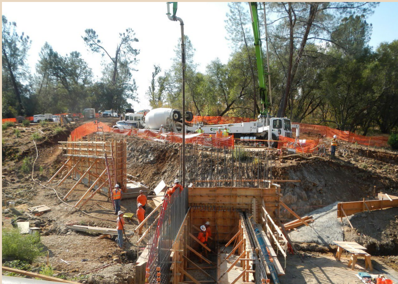
A contractor pours concrete for a fish barrier wall placement at the Baldwin Creek Fish Barrier.
