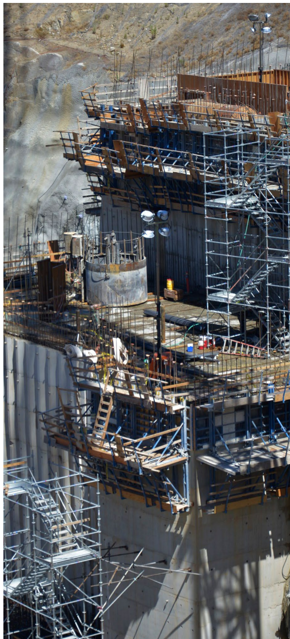
Above and at right, workers construct the auxiliary spillway at Folsom Dam.
