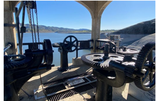
Orland Unit Water Users Association completed the dam's replacement regulating gate installation and the lower and mid-level gates' rehabilitation last fall (its machinery is shown in this photo).
