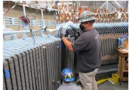
Contractor employee installing one of the 228 new multi-turn coils into the slots in the new stator as part of the Jones Pumping Plant Unit Rewind Project. The C.W. “Bill” Jones Pumping Plant operates in conjunction with the nearby Tracy Fish Collection Facility to protect and salvage fish from pump operations.
