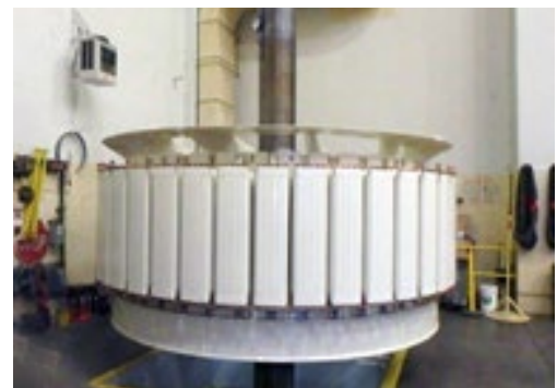
Refurbished unit rotor ready for installation; work included removal of the 40 field pole assemblies, asbestos abatement, windings’ re-insulation, amortisseur bar replacement, and refurbished pole assemblies’ re-installation.
