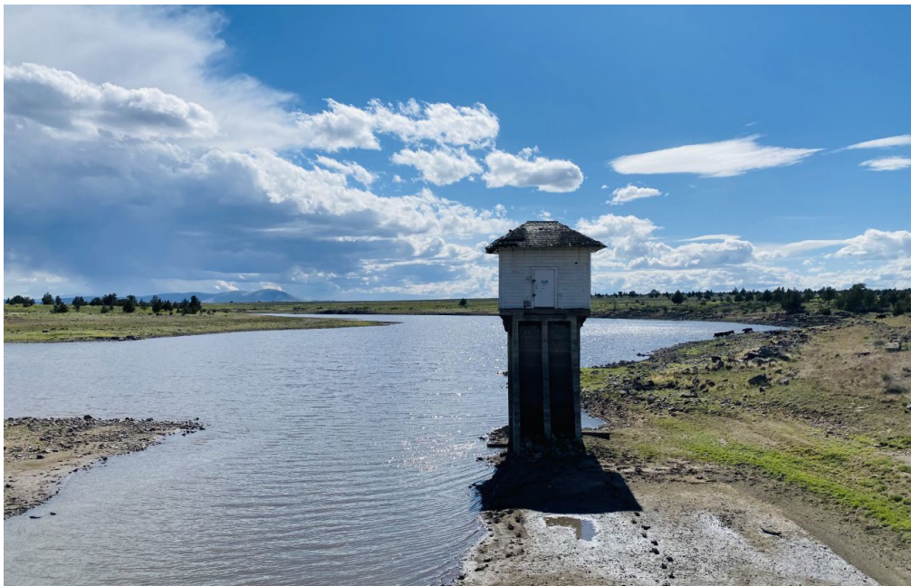
Part of the original dam structure completed in 1910 at Clear Lake Reservoir in Modoc County, California; its levels are reflective of last year's second driest year on record.
