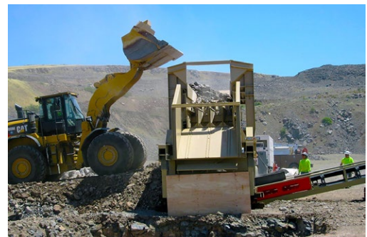
A front loader in action at Basalt Hill Rock Quarry for this Safety of Dams' project near Los Banos; this dam impounds San Luis Reservoir to provide water to communities, farmland, and Pacific Flyway wetlands south-of-the-Delta.
