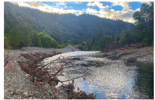
Looking upstream in a new meander constructed on the mainstem Trinity River at the Chapman Ranch Phase B Channel Rehabilitation Project restoration site. Trees with rootwads are buried in the bank to provide stability while riparian vegetation grows in.
