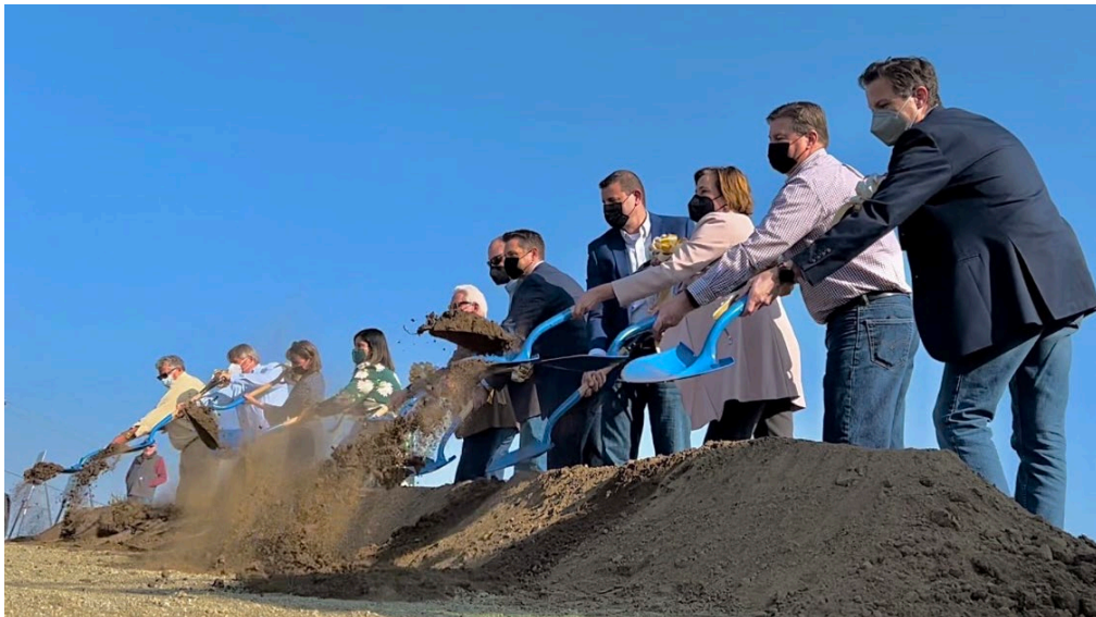
Representatives from the Bureau of Reclamation, Friant Water Authority, California Department of Water Resources, and other partners shovel the project's first dirt at the $500 million Friant-Kern Canal Middle Reach Capacity Correction project site in Tulare County on Jan. 25, 2022.
