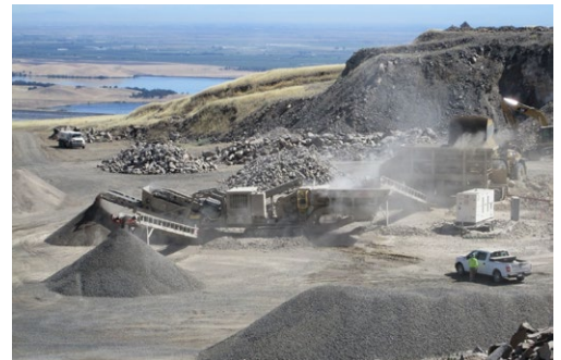
Aerial view of Basalt Hill Rock Quarry next to B.F. Sisk Dam. The front loader places excavated materials in the portable rock screening plant, that material's fed to the rock crusher, and then it is stockpiled via conveyor belts.
