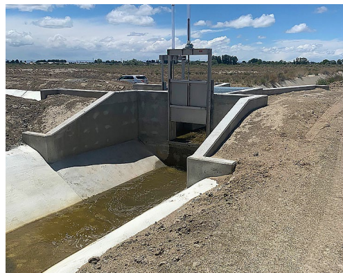
A Fallon Paiute-Shoshone Tribal grant in west-Central Nevada improved and expanded a Reclamation canal within the Reservation. Photo shows a 4-foot stainless steel slide gate at Segment 1 in May 2021.
