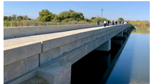
SJRRP completed construction on the Mowry Bridge to improve construction access for the Reach 2B and Mendota Pool Bypass Improvement Project near Mendota in Fresno County.
