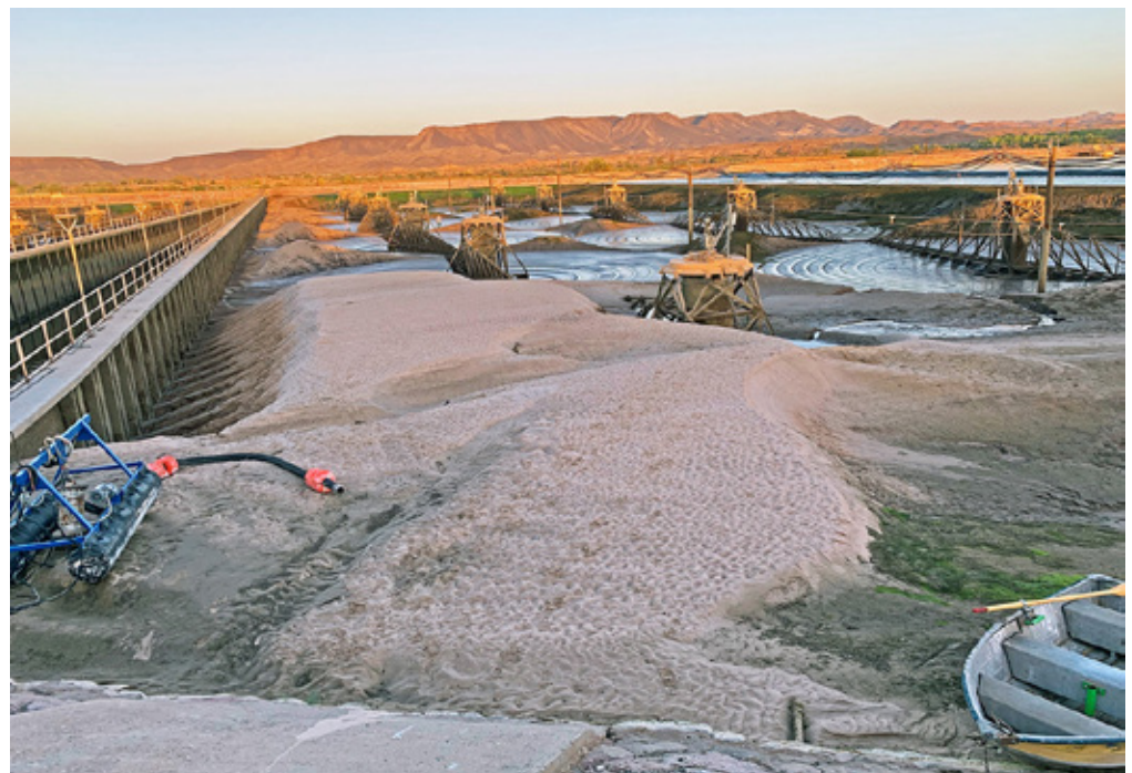
Heavy sedimentation in Basin 3 of the All American Canal desilting works has required sediment removal with heavy equipment.
