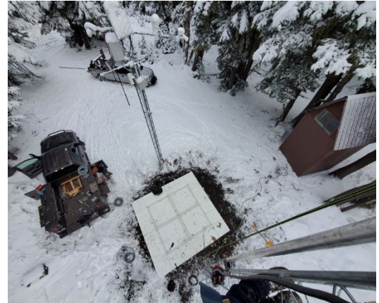
Natural Resources Conservation Service (NRCS) Oregon Snow Survey staff installing an experimental fluidless snow pillow.
