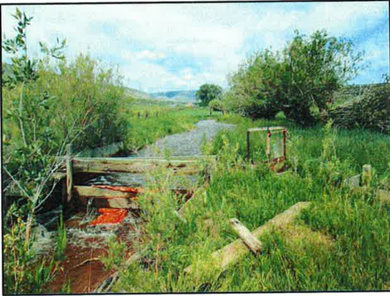
Photo 3: Looking upstream (westerly) at the existing diversion structure that feeds the Cedar Hollow lateral from Birch Spring Draw. This structure is planned to be replaced within the same footprint.
