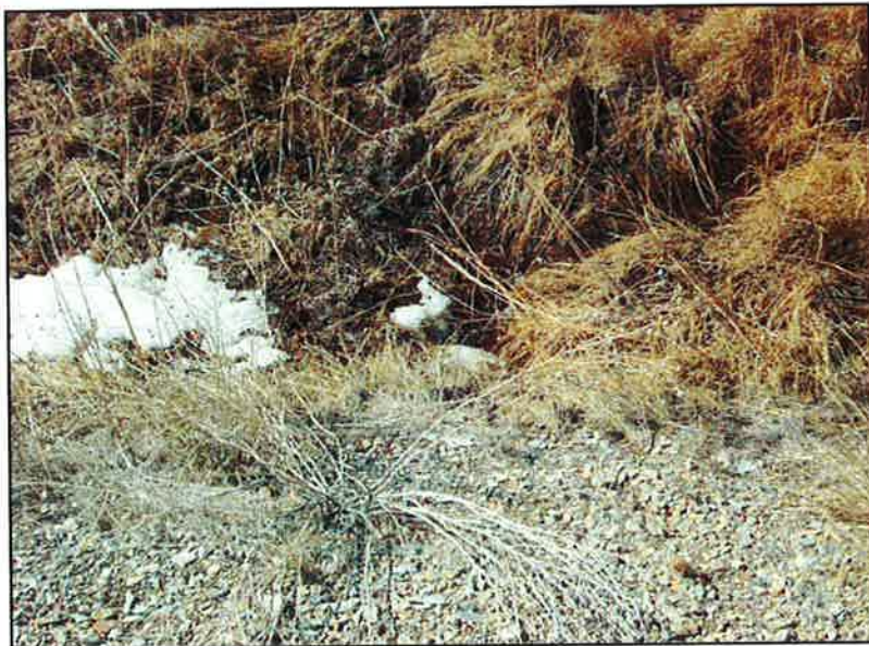
Photo 6: This photo shows the 12-inch outlet pipe that is located at the south end of the HRS. This pipe traverses through Bennion Lane. No modifications are proposed to this pipe.
