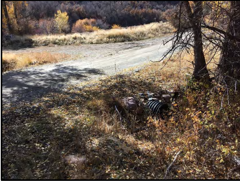
Photo 3: This photo shows an existing drainage culvert that runs under Hardscrabble Road near the existing reservoir.
