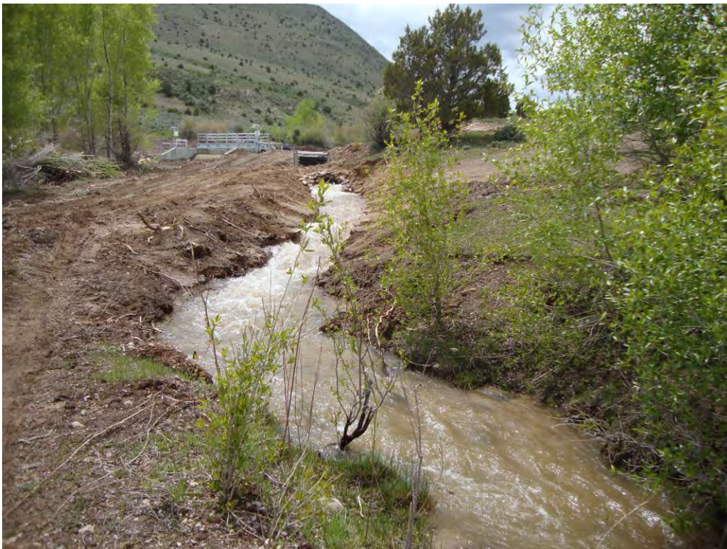
Photo 5. Looking west towards the west terminus of the North Lateral, with the creek diversion structure in the background.
