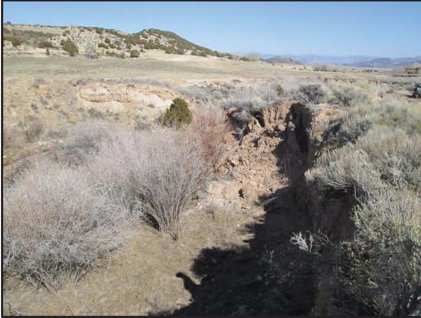
Photo 5: Looking easterly at the right bank of Birch Spring Creek. This near vertical bank is actively sloughing.
