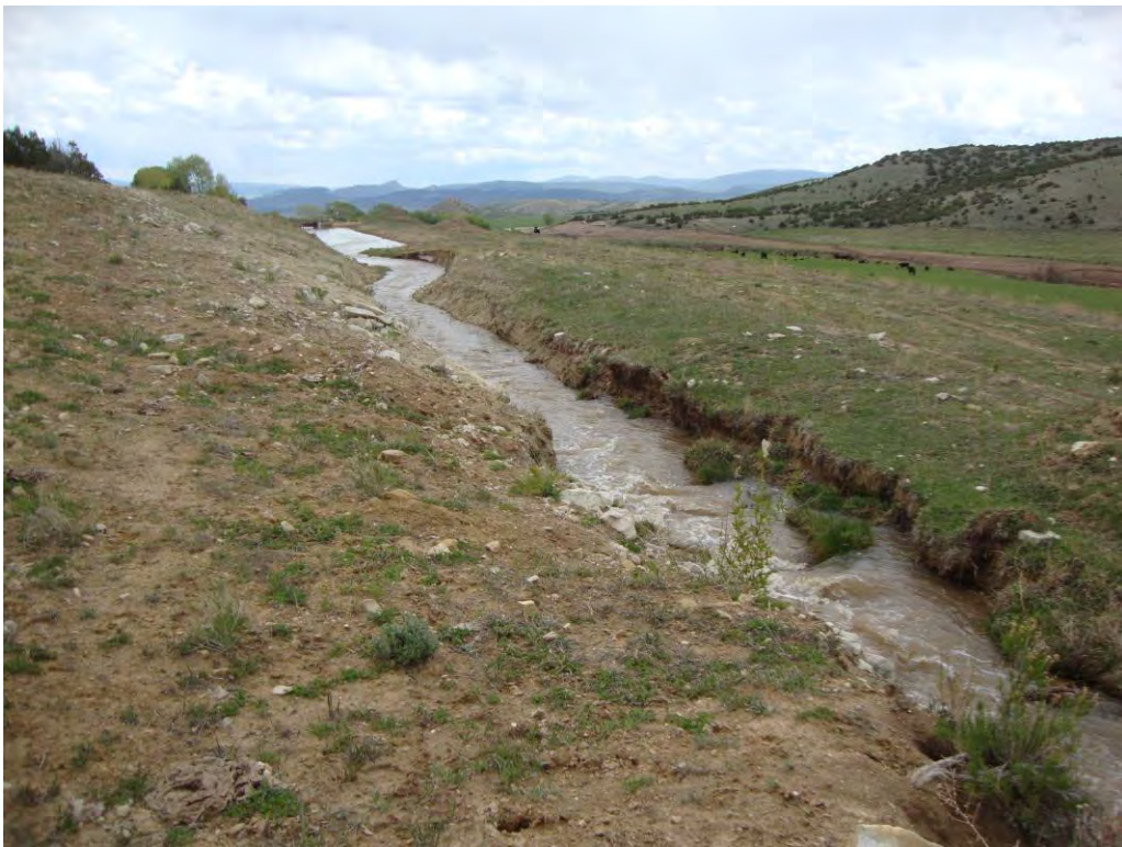
Photo 7. Disturbed section of the North Lateral upstream of the Pallensen Pond in the background, looking east.
