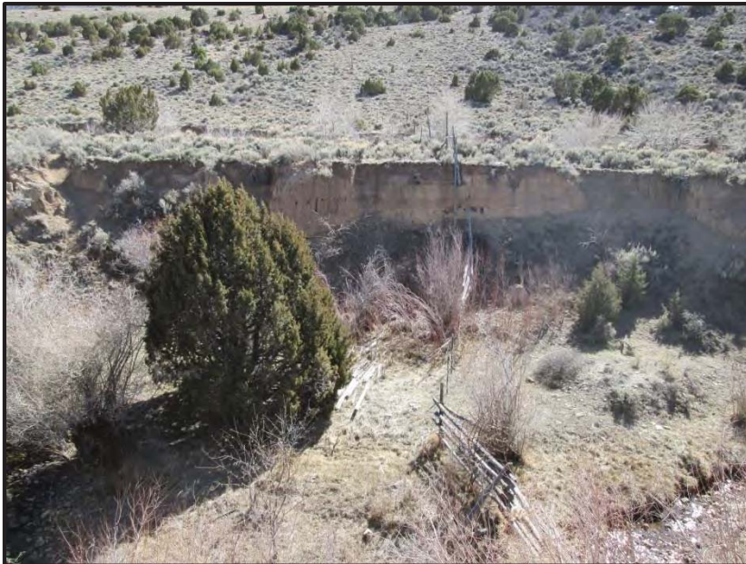
Photo 2: Looking southerly along the western boundary of the Habitat Replacement Site (HRS). A large percentage of the banks of Birch Spring Creek within the HRS are very steep (i.e. near vertical slopes). The proposed earthwork above the OHWM of Birch Spring Creek is intended to lay the slopes back, which will help to stabilize these banks and minimize unraveling.
