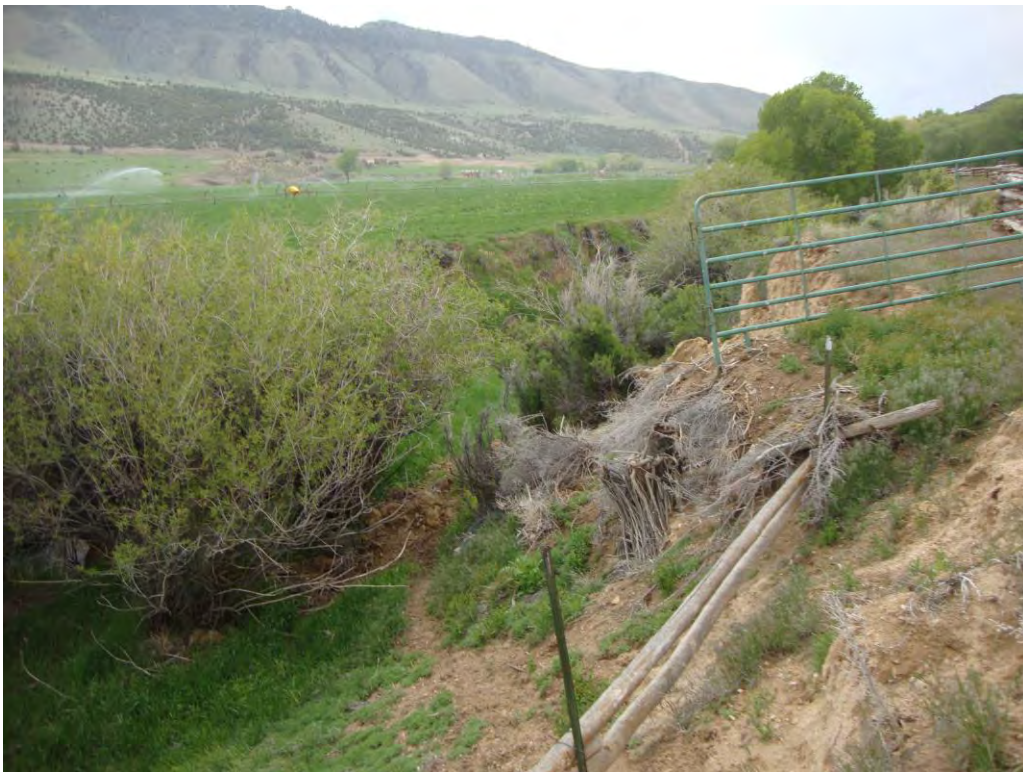
Photo 9. Section of the North Lateral in a large, eroded gully shortly before the east terminus, looking west.
