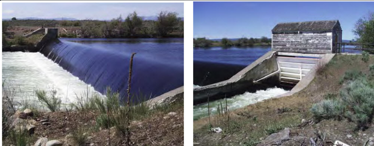
Figure 12. Cross Cut Diversion Dam and radial headgate on the Henrys Fork River.
