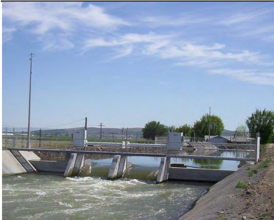
Figure 29. Photo of an automated canal system with a Langemann gates structure.
