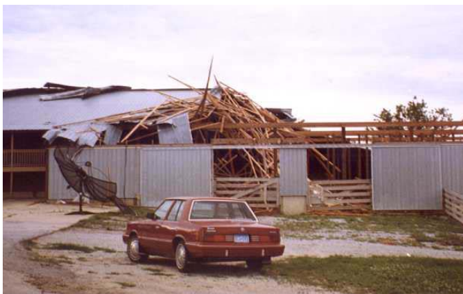
(Wind damage to buildings in southern Minnesota – June 1998)
