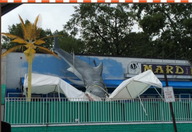
Above: Wind Damage to the Mardi Gras in Cranston, RI. Picture by John Buco.
