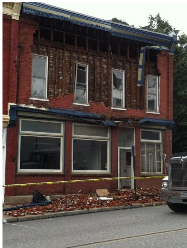
Building Damage – Union City
