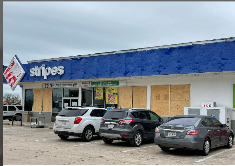
Figure 4: Extensive Damage to a Stripes Gas Station in D'Hanis, TX. Photo by NWS Austin-San Antonio
