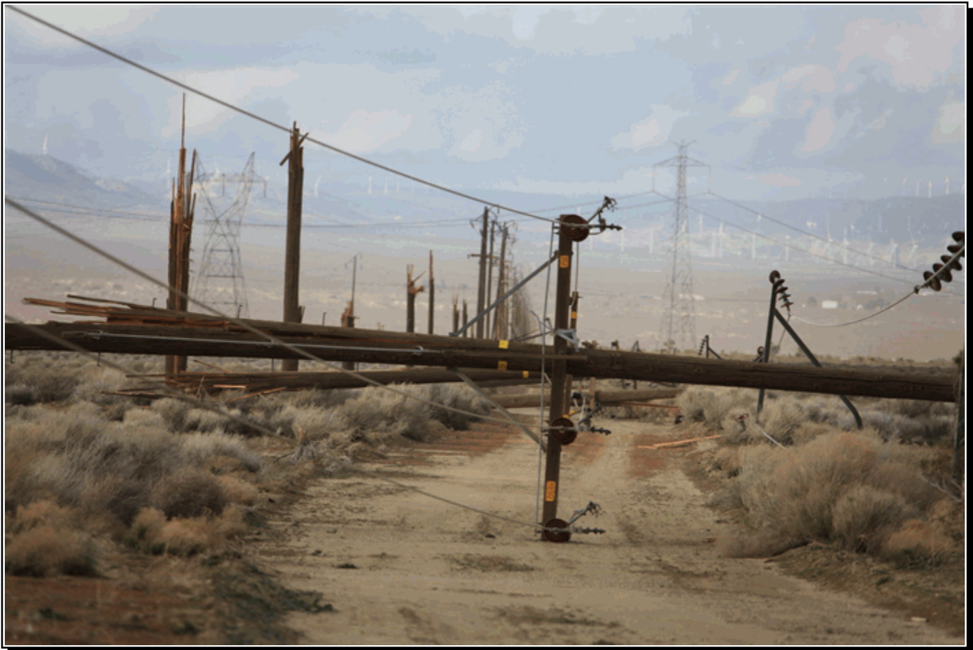
Wind damage from high winds up to 80 mph on March 7th in the Kern County desert. Images courtesy So Cal Edison.
