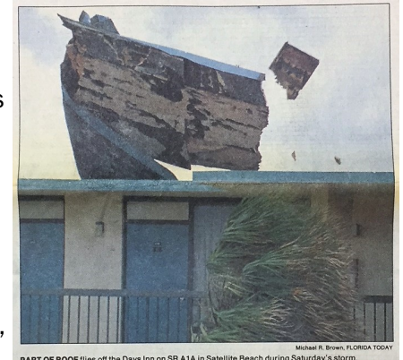
PART OF ROOF flies off the Days Inn on SR 1A in Satellite Beach during Saturday's storm.
