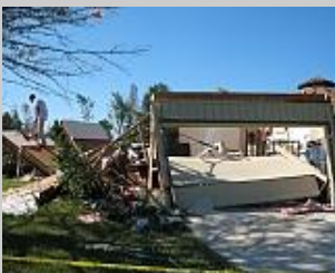
F1 damage to home in Seminole County
