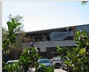
F0 damage to warehouse in Seminole County
