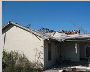
F1 damage to home in Seminole County
