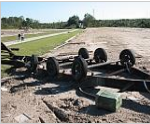
Completely demolished mobile home (unsecured) in Seminole County
