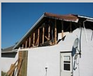
F0 damage to home in Seminole County
