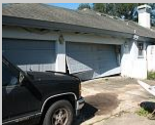
F0 damage to home in Seminole County
