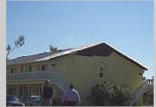
F0 damage to apartment building in Orange County.
