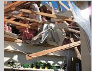
Damaged interior of home in Seminole County
