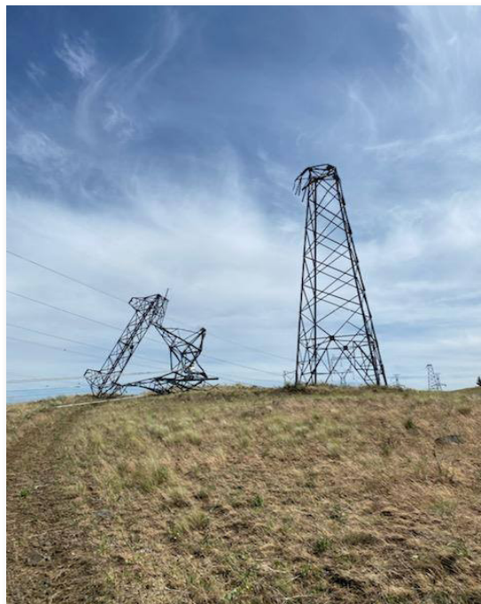
Damage from severe thunderstorm winds on exposed power line tower near Shaniko, OR.. Photo by Erik Pytlak, Bonneville Power Administration.
