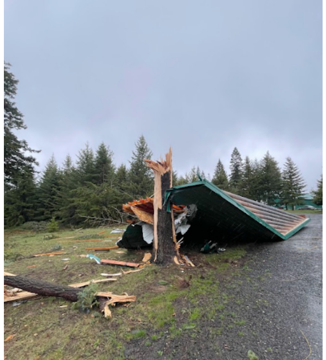
Figure 7 Uplift of roof deck with loss of roof material indicative of EF1 damage. Photo taken by NWS Employee.
