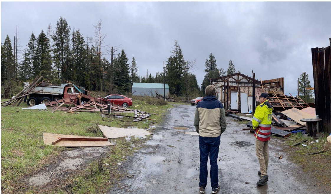
Figure 8 Collapse of farm outbuilding walls. Shown are NWS Employee Brandon Lawhorn (left) and East Umatilla Fire & Rescue Chief Dave Baty (right). Photo taken by NWS Employee.
