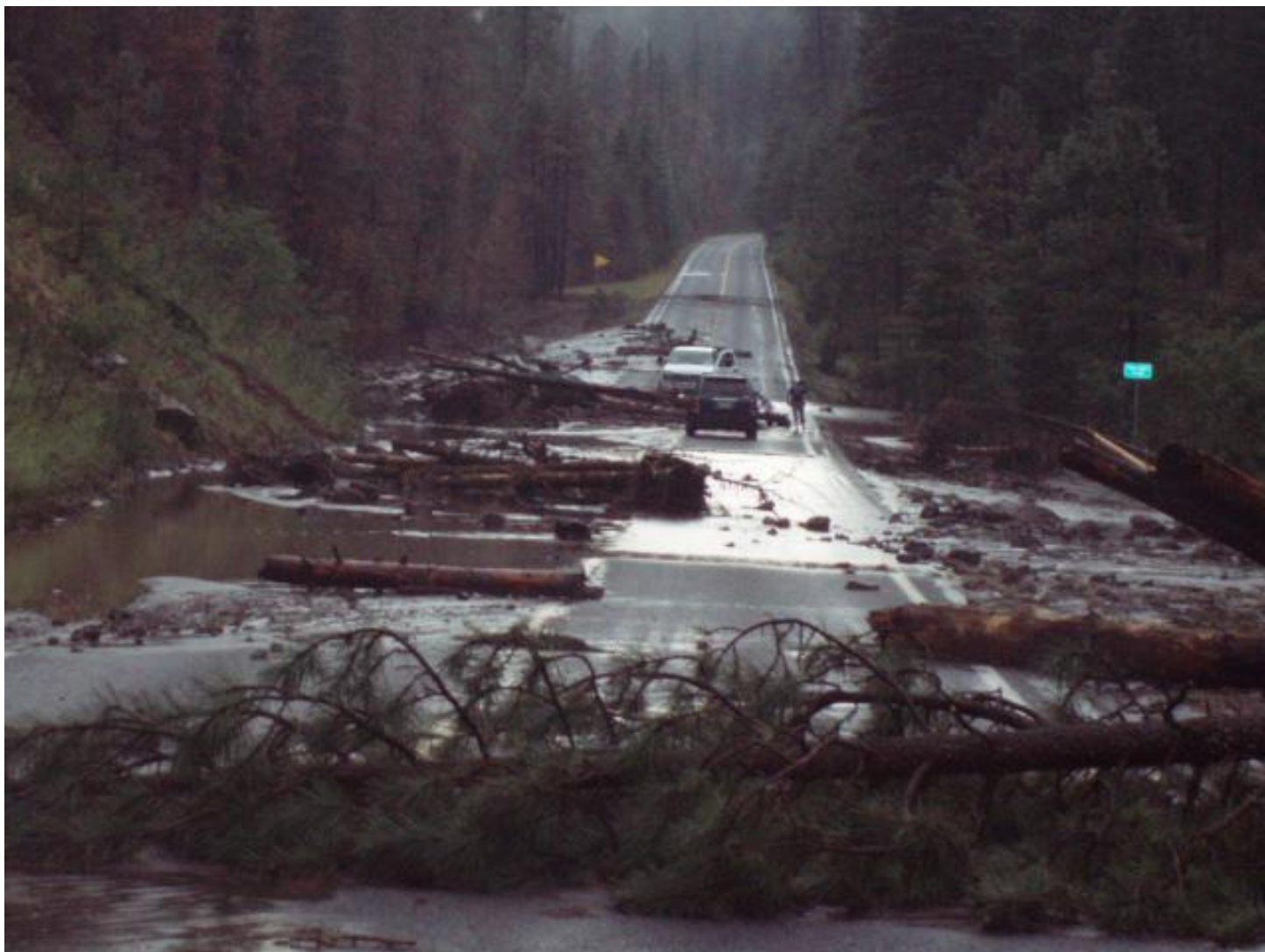
Figure 79. Hannagan Creek Basin at Highway 191 (photo provided by AZDOT). Culvert became blocked and Hannagan Creek flowed over Highway 191. Flow was 4-8 feet deep over road above culvert (near where person is standing in photo). Perpendicular to direction of flow, from highwater mark to highwater mark, was a distance of 980 feet (in photo you can see far highwater mark near yellow sign). The highwater marks were likely not made at the same time. Also, the flow across the road may have at times been braided or the direction of flow may have not always been perpendicular to the road. Cross Section #2; Main watercourse over road estimated as 30 feet wide, 6 feet deep, having a shape of half an ellipse, a wetted perimeter of 36 feet, a n value of 0.055, and a slope of 0.022. Estimated flow = 1,405 cfs. Mean velocity = 10 ft/sec. [Estimated flow = 1,360 cfs using a broad crested weir equation 24 with hydraulic head (H) = 6 feet, weir length (L) = 30 feet, and discharge coefficient (C) = 3.09.]
