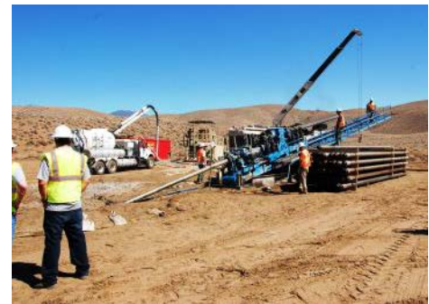
NTIA staff met with the crew at a California Broadband Cooperative construction site in Inyo County, California.
