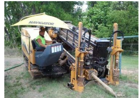
A member of a Peoples Telephone Cooperative construction crew installs fiber in Canton, Texas.
