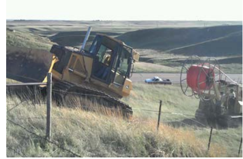
A NebraskaLink construction crew prepares to install fiber at a site in Imperial, Nebraska
