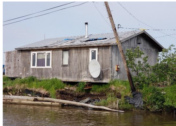
Home affected by permafrost and erosion and that is a first priority to move away from the riverbank. However, it cannot be moved due to an unstable foundation.
