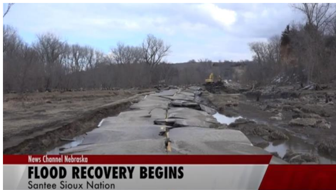
Highway 12 at the western edge of the Santee Sioux Reservation. Road completely destroyed by the flooding of 2019.
