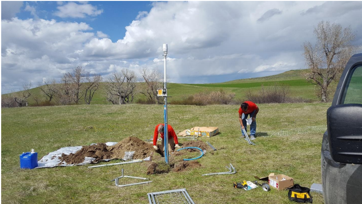
Figure 10. Installing a weather station near Crow Agency, Crow Reservation, as part of a statewide program to provide local weather data for short-term uses and long-term climate adaptation planning.
